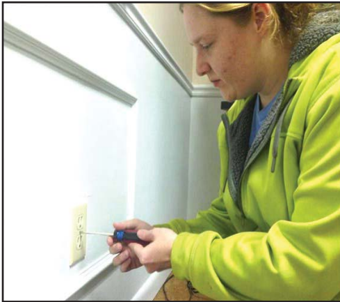
Jeri Daugherty works on an outlet in the Marion County Senior Citizens building.
